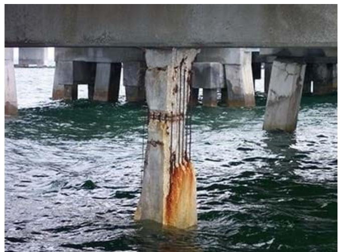
Concrete column damaged by saltwater
