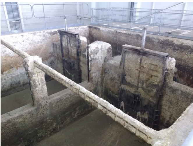
Concrete surface eroded by H 2 S Hydrogen Sulphide
